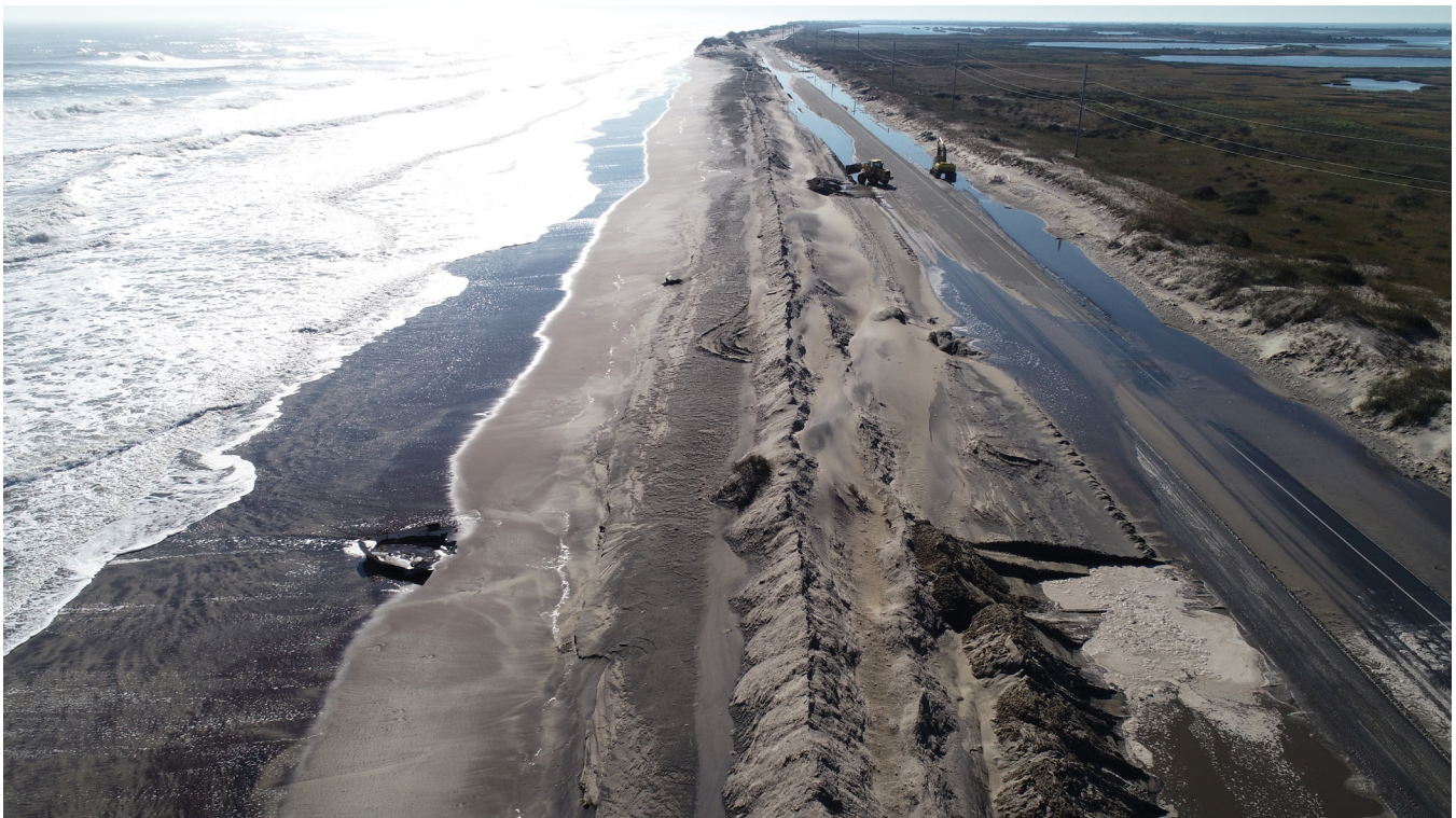
NC 12 Flooding at the Canal Zone Hot Spot after November 11, 2021, Coastal Storm
