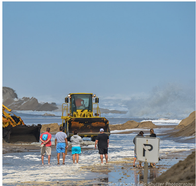
Closure and Emergency Repair of NC 12, September 22, 2020
