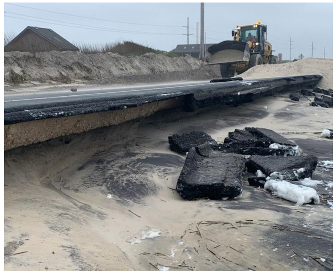
PINWR Visitor Center Road Washout, May 5, 2022
